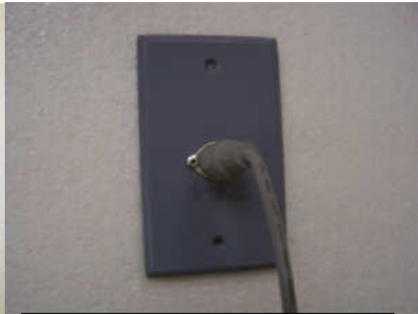
Cable – Junction Box Receptacle
